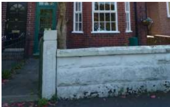
Original stone wall and gatepost at No. 10 paving Weldon Road, though this example has been painted inappropriately
