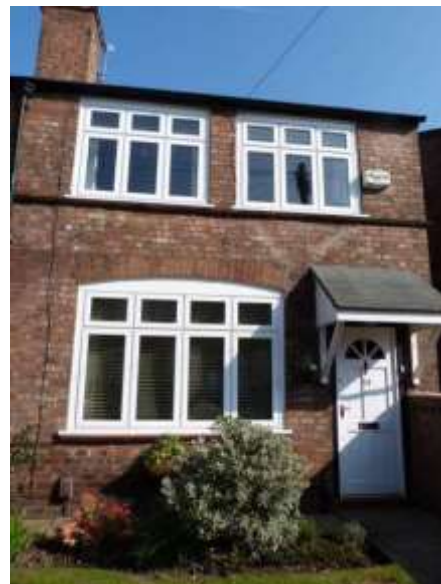
uPVC windows which are a more successful example, though with thicker frames than the original, at No. 14 Place Road
