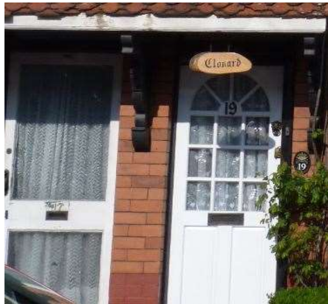
Inappropriate replacement doors to Nos. 17 and 19
