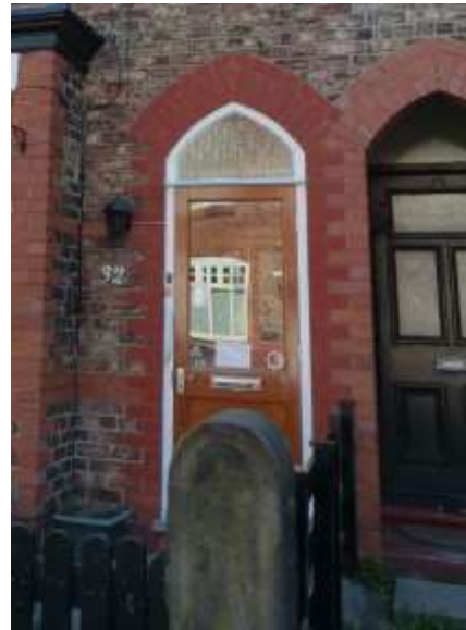
Inappropriate door at No. 32 Weldon Road in stained timber, which is set forward with the loss of the original porch
