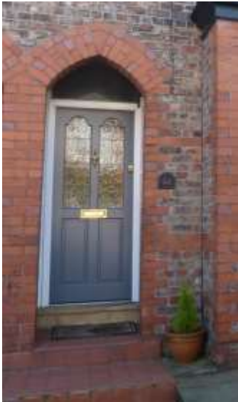
Door at No. 34 Weldon Road, which follows roughly the original design, using timber and glazed upper panels, but which does not exactly follow the original style and would therefore not be permitted in any future applications
