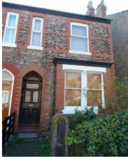
Appropriate timber sash windows on the ground floor of No. 30 Weldon Road, though the first floor windows are inappropriate uPVC replacements
