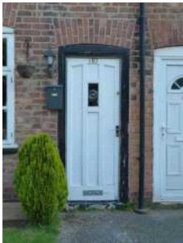
Timber framed door but not in the original style at No. 107 Lawrence Road
