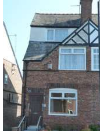
Inappropriate windows at No. 53 Lawrence Road
