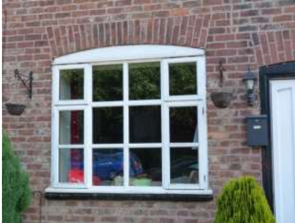
Inappropriate windows at No. 107 Lawrence Road
