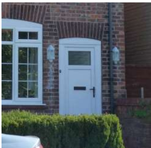
uPVC door in the original style at No. 63 Lawrence Road but with a chunkier appearance than the timber versions
