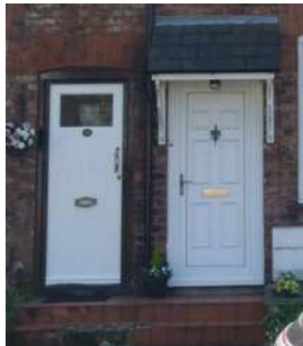
An inappropriate uPVC panelled door (No. 13 Bemrose Avenue, right) with modern porch next to an original timber door (No. 11 Bemrose Avenue, left)
