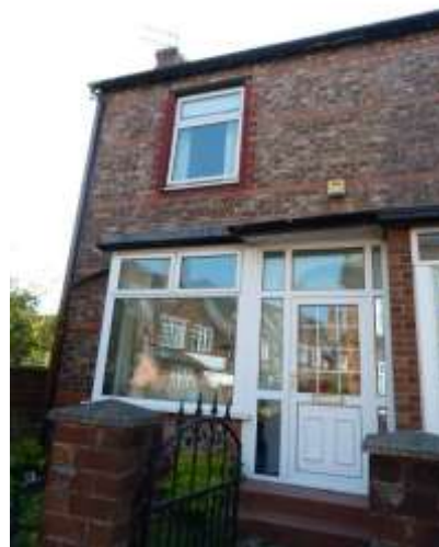
Inappropriate porch and uPVC windows at No. 48 Weldon Road
