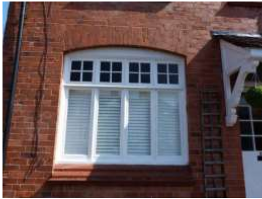
Style Six: Original window featuring coloured glass panes on No. 57 Lock Road
