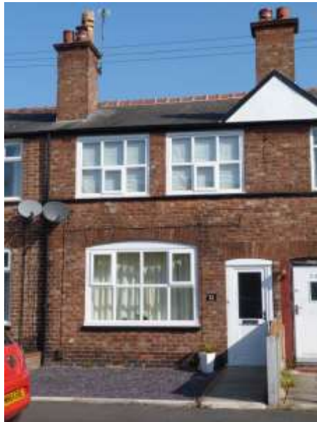
Inappropriate windows at No. 22 Place Road, which have the wrong frame composition. Note also how the top hung casements project outwards from the main frame, increasing the thickness of the frames and disrupting the smooth lines of the frame
