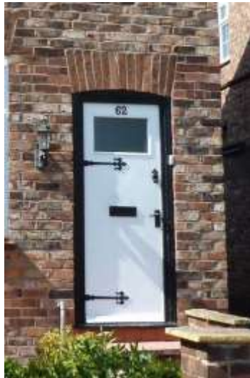
Original door at No. 62 Lock Road, though the decorative ironwork is not original and is inappropriate
