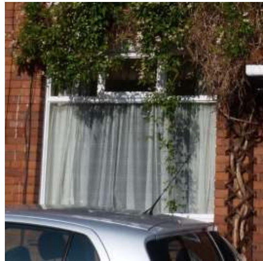
Replacement window at No. 5 with the incorrect composition
