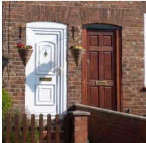
Inappropriate doors on Place Road
