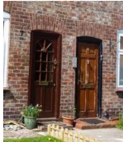
Inappropriate doors on Lock Road
