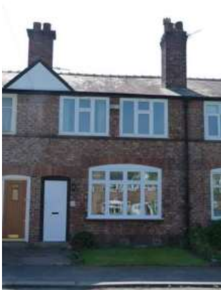
Replacement timber windows at No. 25 Bemrose Avenue. These are timber frames. The ground floor window has the correct frame design but the first floor windows lack some of the smaller upper panes. The frames are also thicker than the original examples
