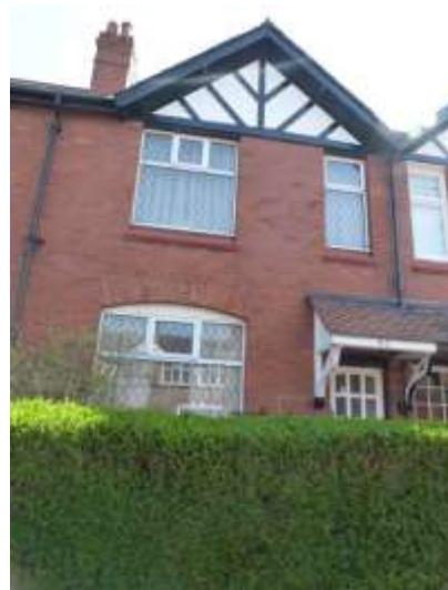
Style Six: Inappropriate leaded windows at No. 51 Lock Road
