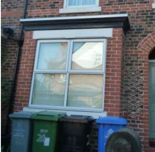
Inappropriate uPVC windows to No. 20 Weldon Road
