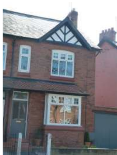
Style Seven: uPVC windows to No. 21 Norman Road which follow the pattern of the original windows but which are bulkier than a timber frame
