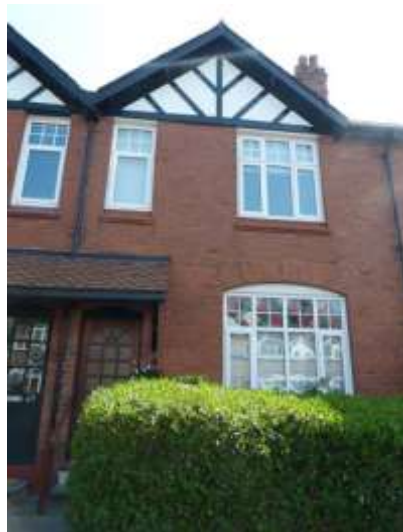
Style Six: uPVC examples of windows following the original design, though with bulkier frames
