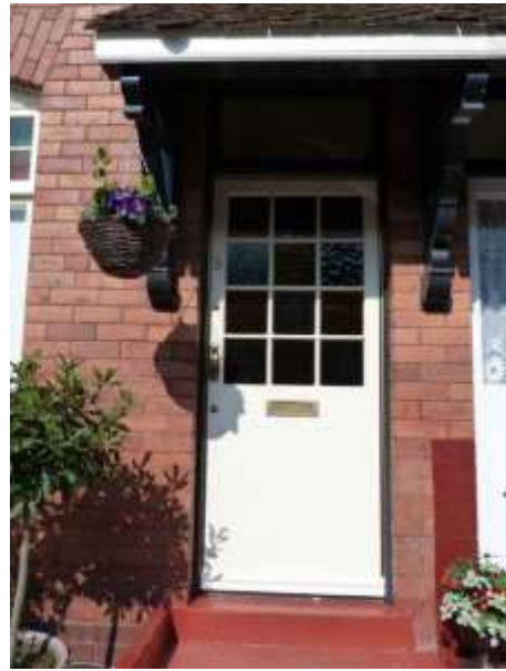
Original door to No. 9. Some of the coloured glazed panes have been replaced with textured glass
